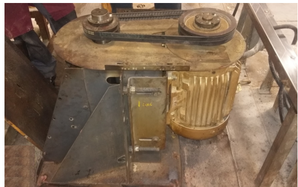
↑ Oven Re-Circulation Fan Unit
